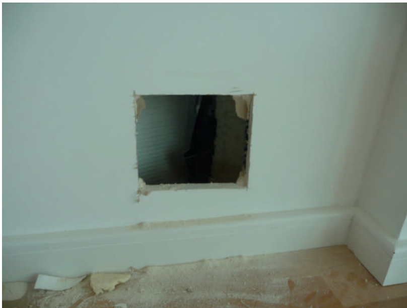
26. Lounge cold area from infra red survey showing missing insulation, vapour barriers etc.
