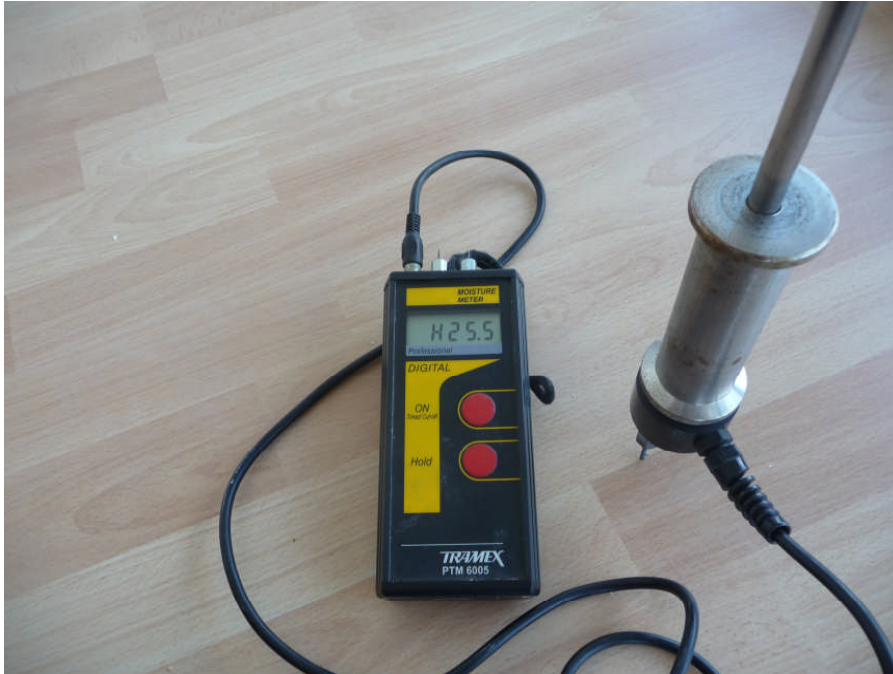
21. Screed shows 25.5% WME at window area of lounge
