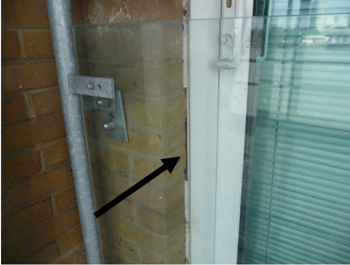
27. Outside view of photo (25- 26 ) showing gaps in brickwork and lack of weatherproofing (sealant)
