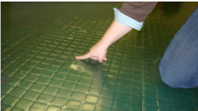
Photograph 9: Failing Vinyl Composition Flooring
