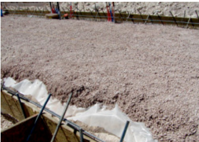
Photograph 2: Slab-on-Grade Done Wrong
