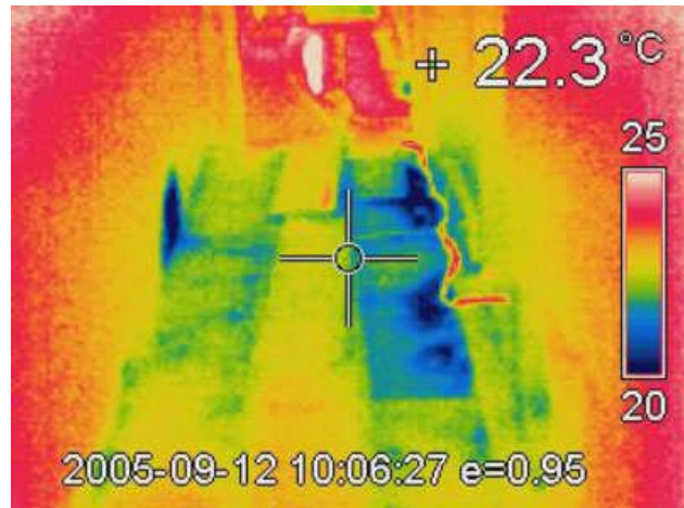
Several sub floor leaks identified from faulty pipe work installation.
